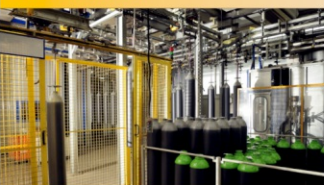
Gas production and bottling
